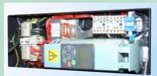
Internal view of electric cabinet with its inverter.
